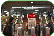
Lifts, escalators &amp; lighting
