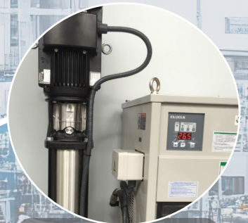
▲ Motors & Drives - Inside machinery
