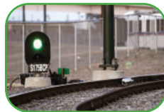
Trackside signal &amp; power
